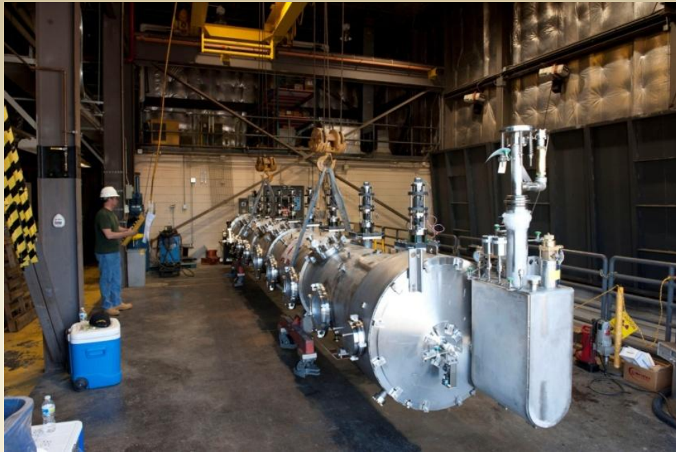
New Cryomodule – staged in Access Building prior to installation in tunnel
