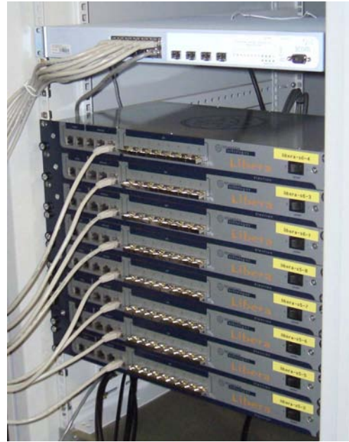
Figure 1: Libera installation for one section of the storage ring
