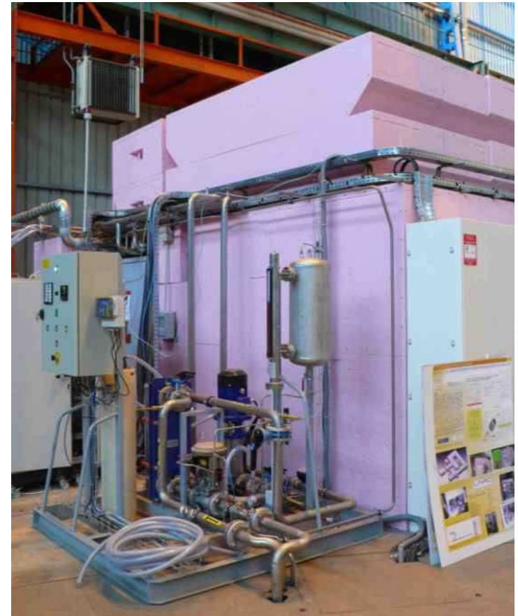
Dedicated water temperature regulation for magnets and linac
